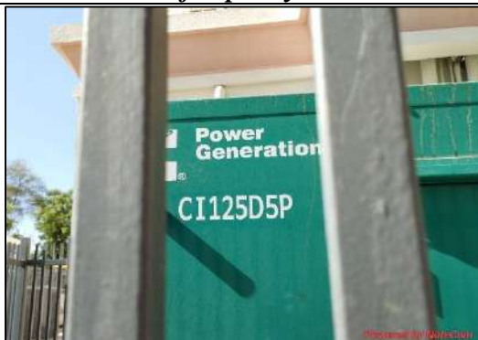
DG Set of capacity 125 KVA
