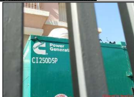
DG Set of capacity 250 KVA
